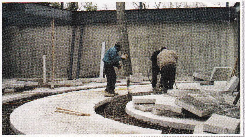
Workers lay the foundation for the Toronto Sportsmen's Show Amphitheatre, part of the new O.F.A.H. |Mario Cortellucci Hunting and Fishing Heritage Centre which is slated to open in the spring.
